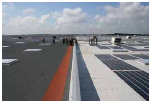
Installation solaire photovoltaïque
